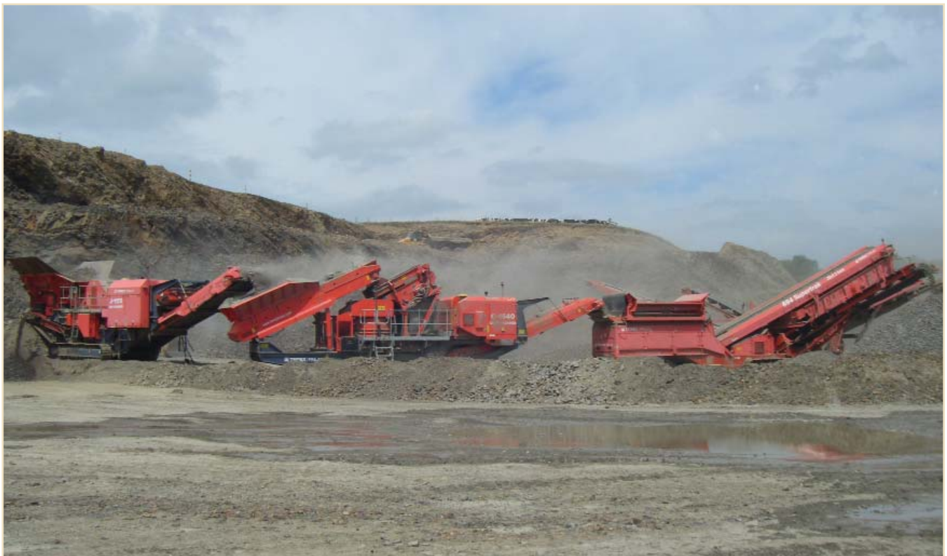
J-1175 Jaw Crusher, C-1540 Cone Crusher, 694 4-Way Screener working in sequence
